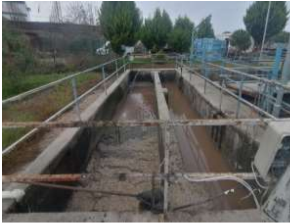
Photograph 12. Aerated Grit Chamber
