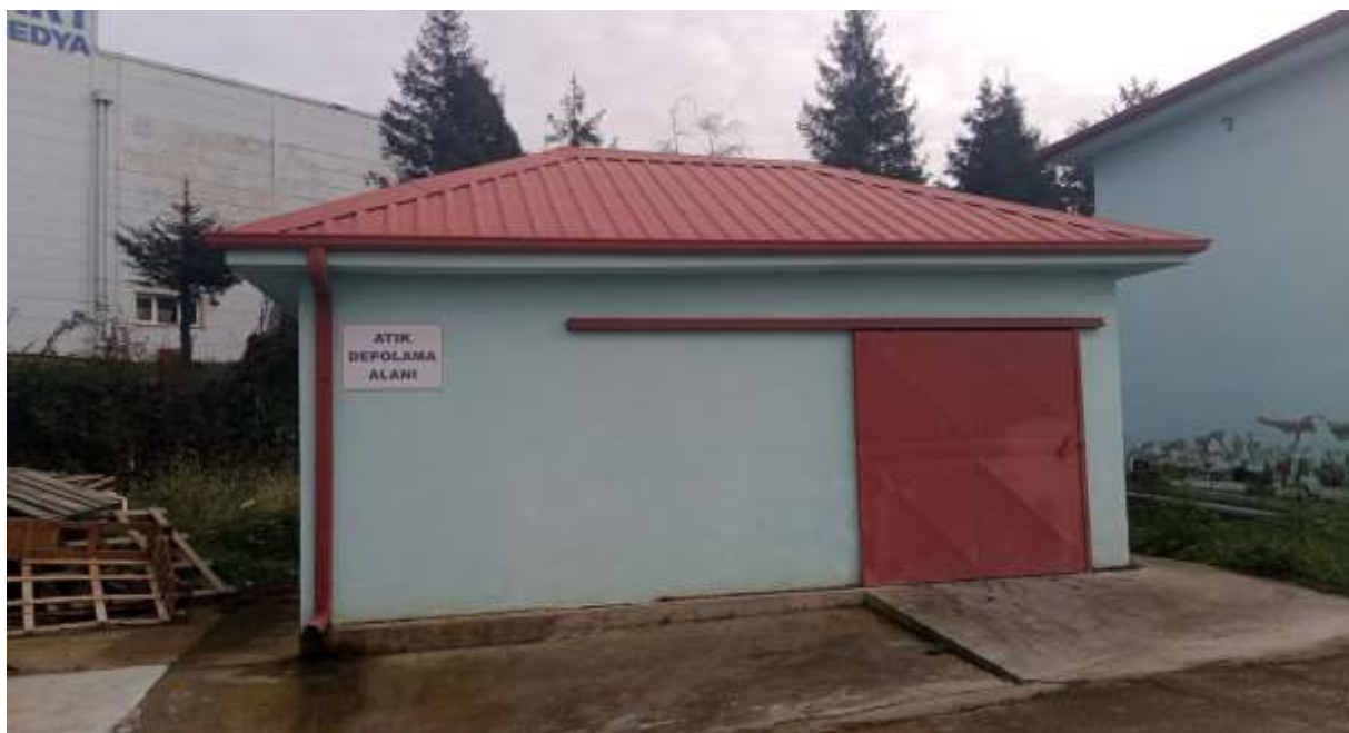
Photograph 18. Hazardous Waste Storage Area
