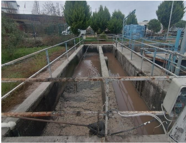
Photograph 12. Aerated Grit Chamber
